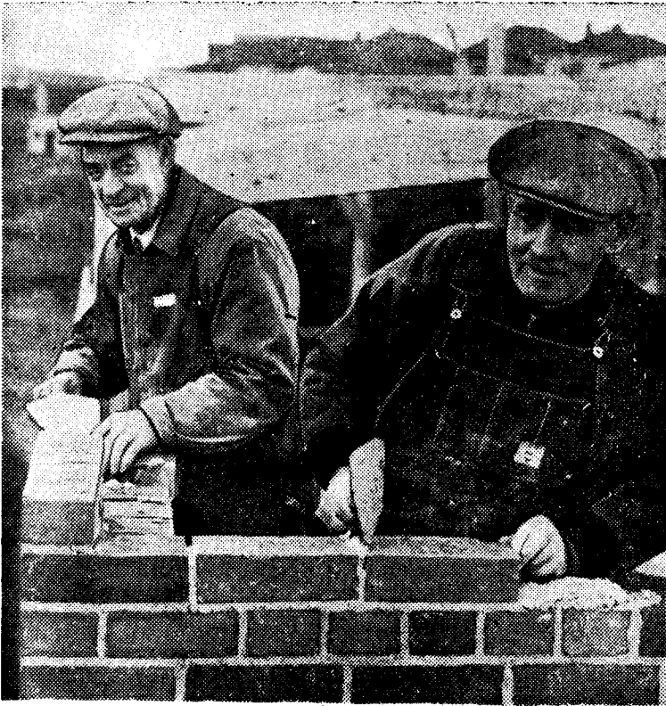
Using the bricks which the volunteers of the Workers' Educational Association produced in their spare time, Bill Mitchell and Jack Henderson, members of the Bricklayers and Tilers local union No. 2 erect the W.E.A. Model Home at Toronto.
